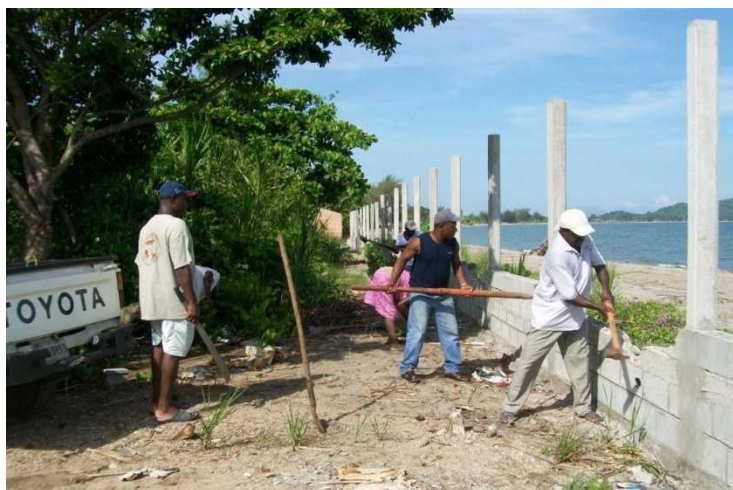
Triunfo de la Cruz community members demolishing an illegal wall. (Photo: OFRANEH)
